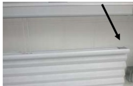
Figure 4: Strike plate on the top of the middle rail.
